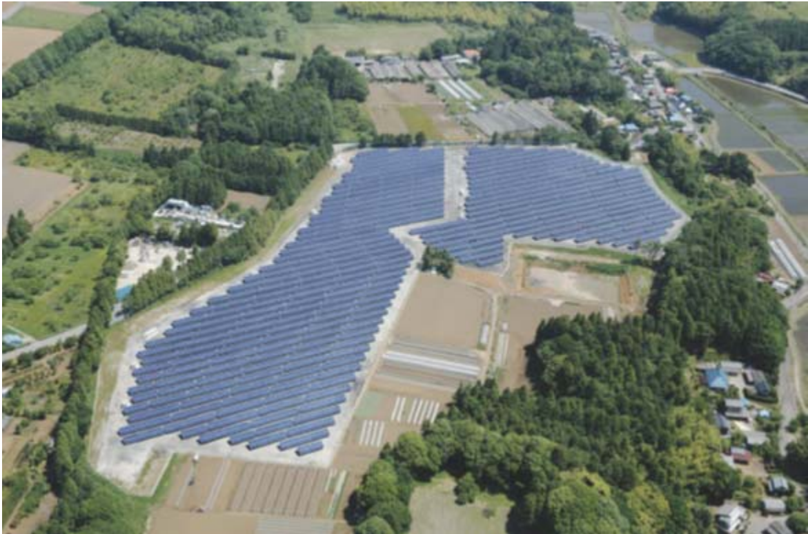
Kasuga Capital Ikazuchi East Solar Plant • Kasuga Capital Ikazuchi West Solar Plant
